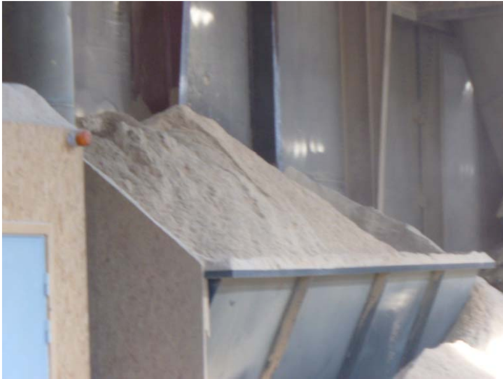
Fig 15. Hopper filled with dust to be made into pellets. Also the walls are not secured
