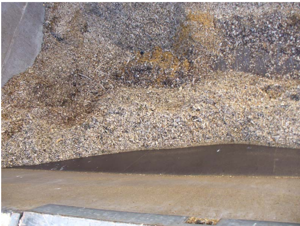
Fig11. Shows the build up of chip on the sides of the hoppers.
