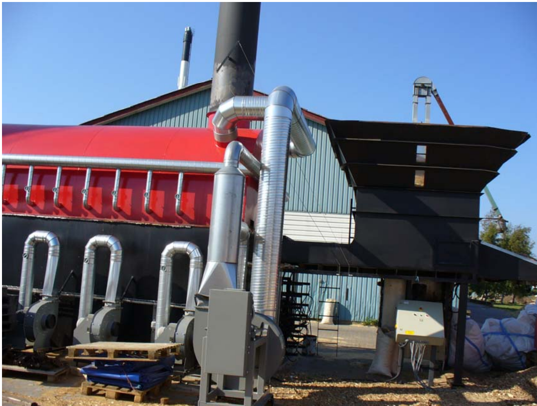
Fig 14. Shows the in feed system to the drier.
